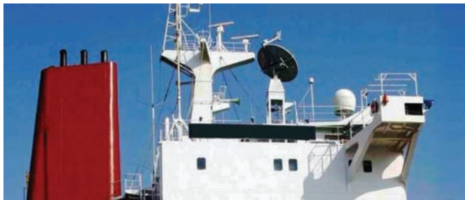
A C-Bird antenna like this one (centre of picture, without radome) survived the 90mph winds of Hurricane Sandy at Maritime Broadband's New York office
