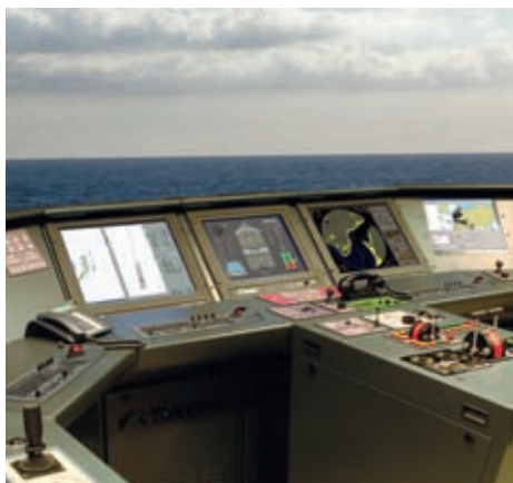
Integrated navigation systems can consist of a number of displays, that can be set up in the optimal configuration required for current operations
