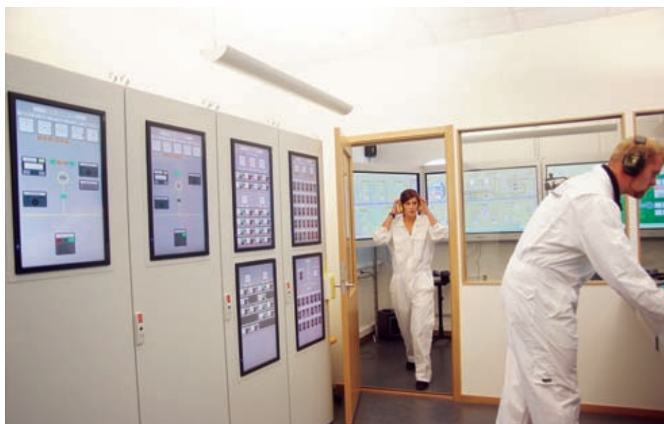
The complete engine room simulator incorporates a number of different simulated systems
